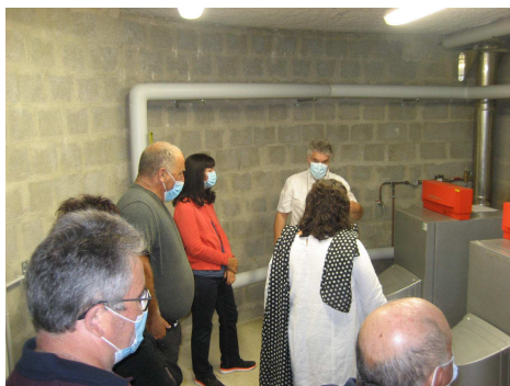
La chaufferie fuel
